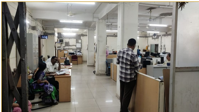
Existing office — damaged ceiling, dated services and worn finishes
