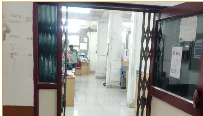
Original entrance — worn flooring and deteriorated wall surfaces
